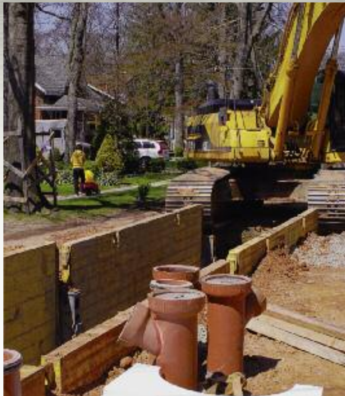
Neighborhood friendly Slide Rail System in action within a Staten Island community.
